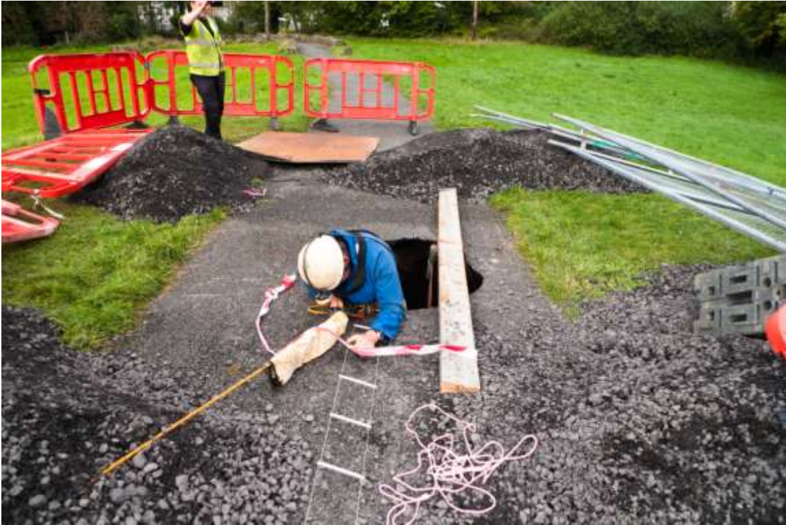
Figure 14. Entrance Shaft which appeared in the footpath in October 2011
