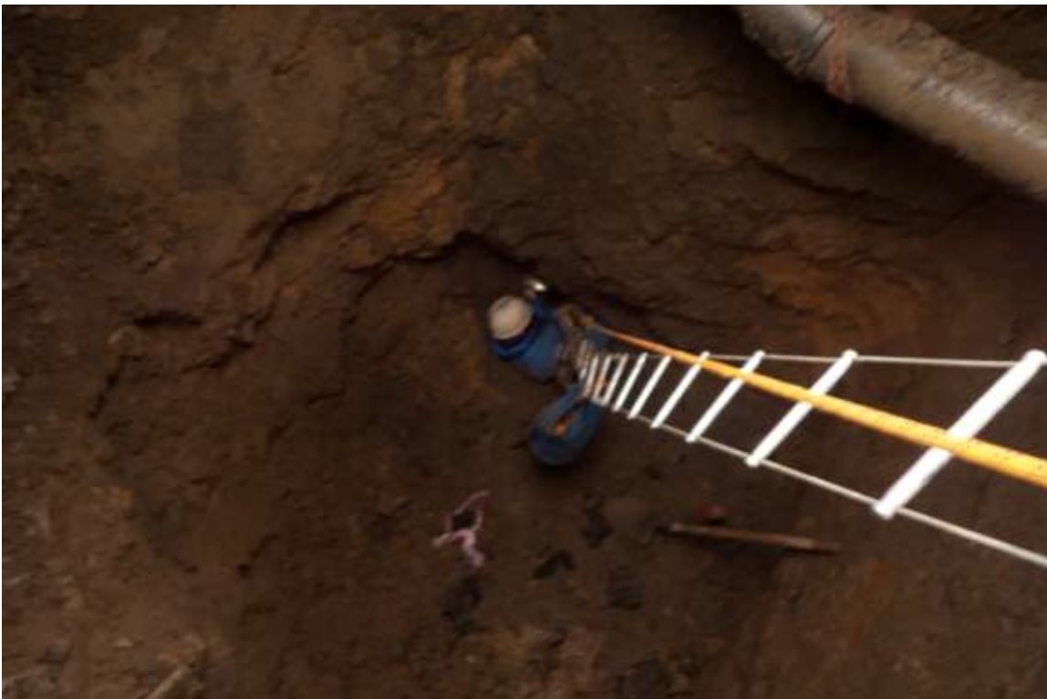
Figure 15. Looking down the entrance shaft showing water main in the top right
