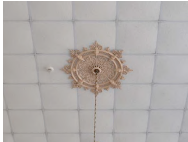
Fig 27: View of suspended ceiling in the courtroom with the original ceiling rose
