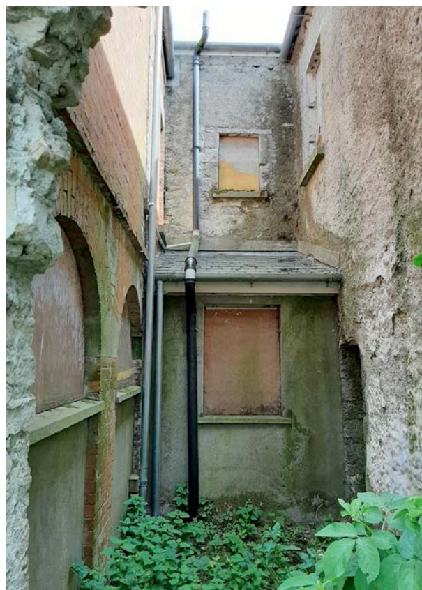
Fig 50: Single storey lean-to shed with asbestos tile roof to the rear of courthouse
