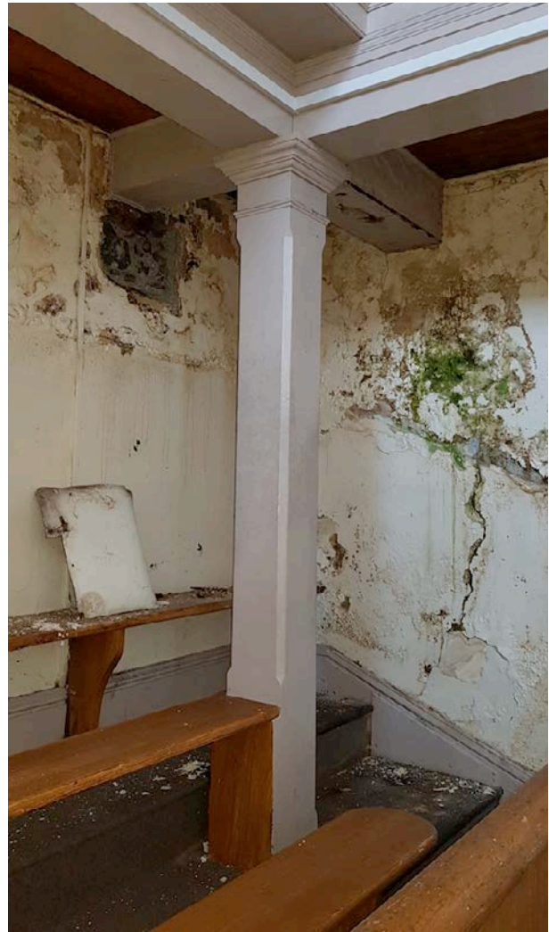
Fig 33: Damage to plaster due to excessive water ingress
