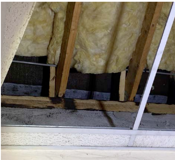
Fig 26: View into roof space over courtroom with concrete ring beam, modern creosoted timbers and blanket insulation
