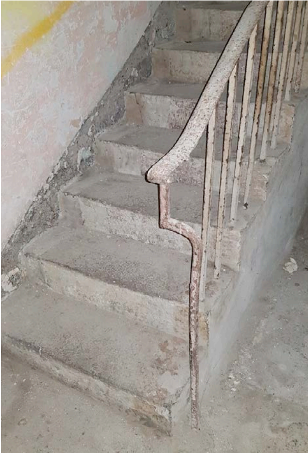
Fig 34: The stone cantilever stair in the south range with rusted handrail
