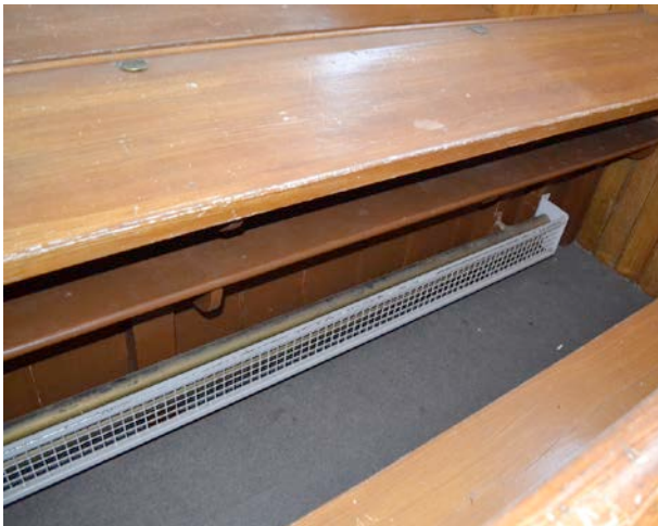
Fig 42: Heating pipes mounted to the back of the courtroom joinery
