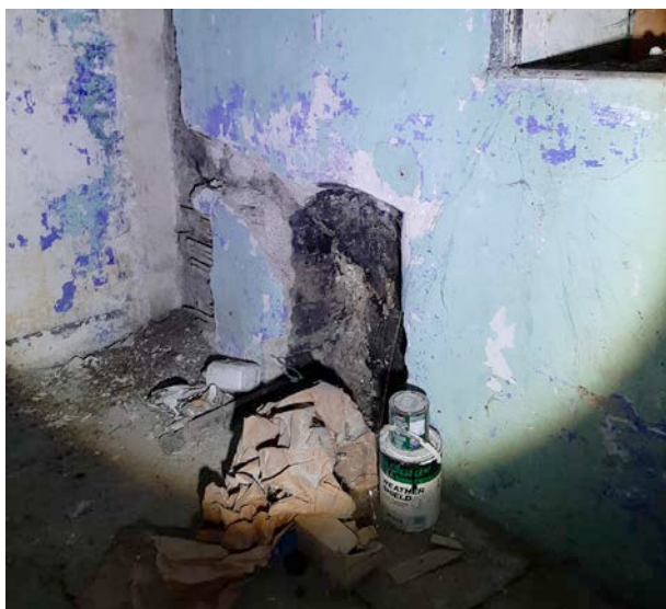
Fig 49: Evidence of continual deterioration in the south range
