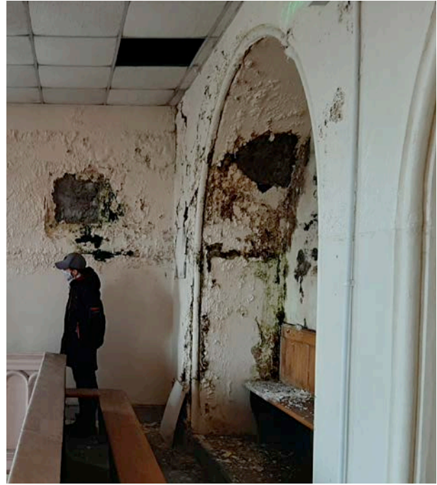
Fig 32: View of damaged plaster on gallery level in courtroom
