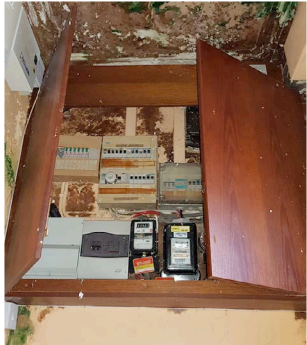
Fig 43: Electrical panel in entrance lobby
