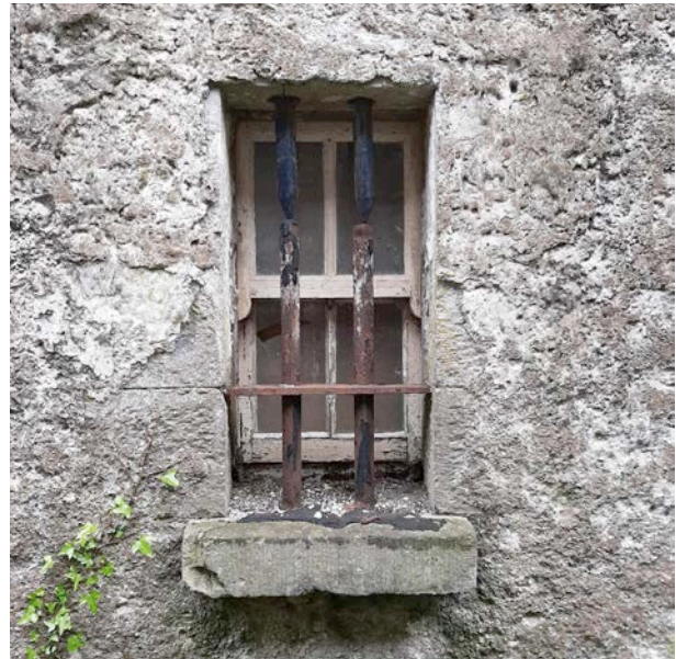
Fig 24: Timber cell window with rusted iron bars in stone sill
