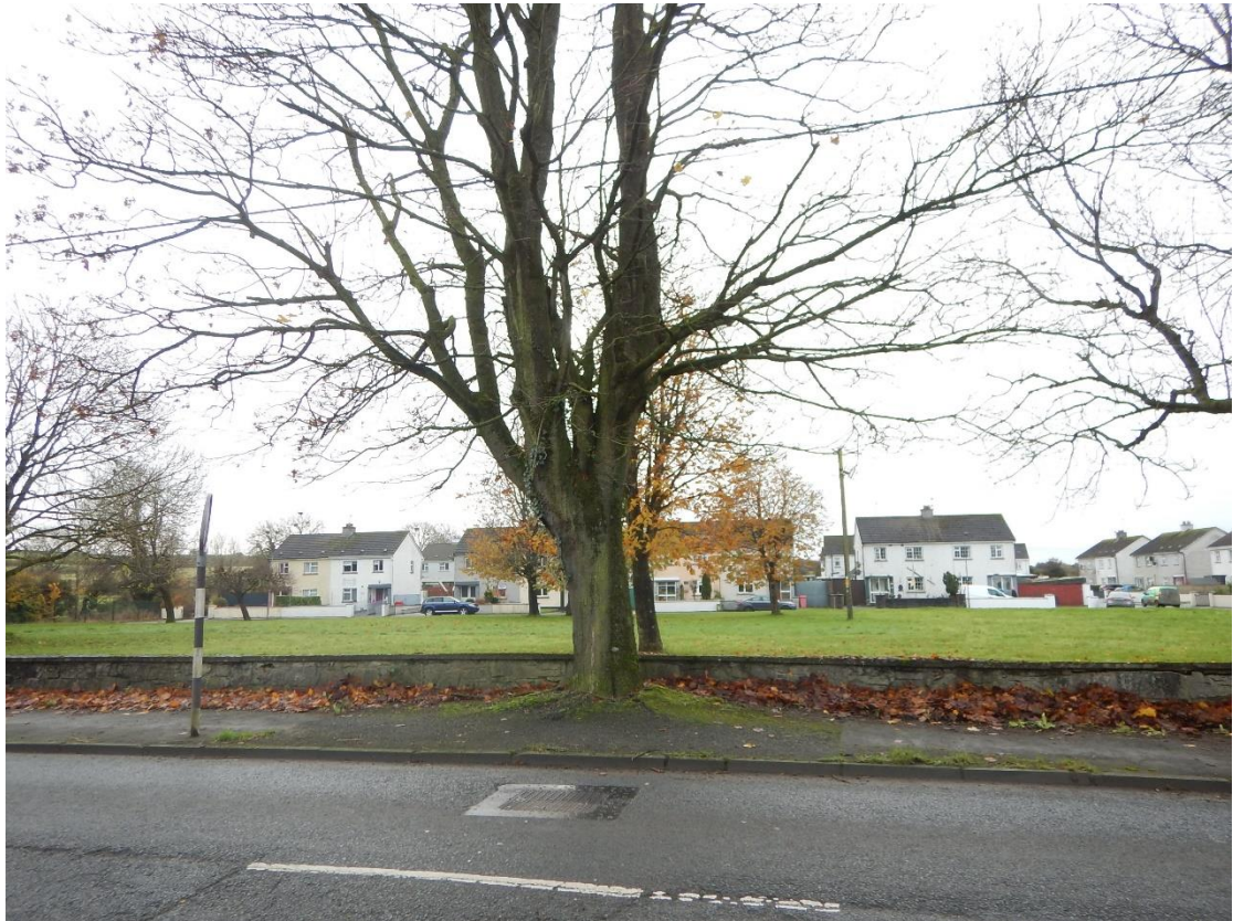
3. Maple tree T754 viewed from the north, with severe distortion of the tarmac surface clearly visible
