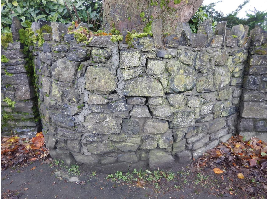
5. Short section of stone wall built around the stem base of Sycamore tree T757, note the significant cracking of the masonry
