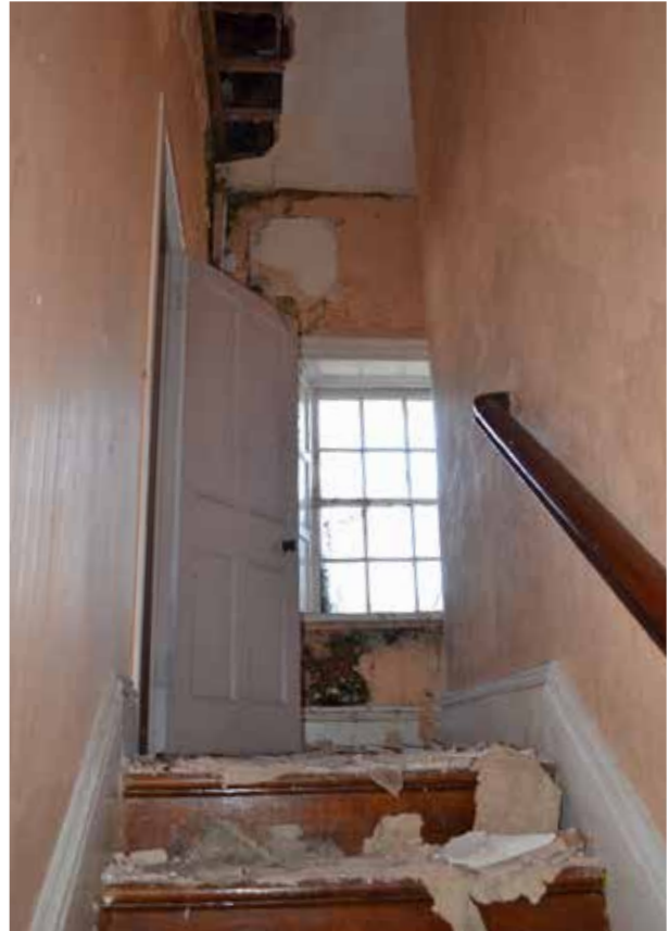
Collapsed ceiling in stairwell, decay around window.
