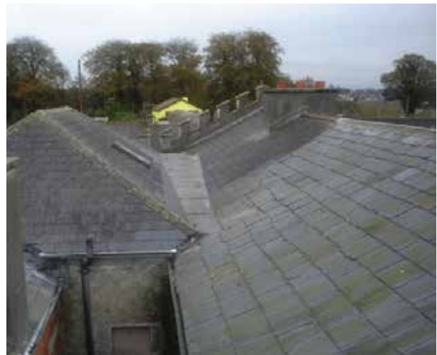
Roof of prison range on right with mix of natural and fibre cement slates. Entrance range roof fully slated in fibre cement slates
