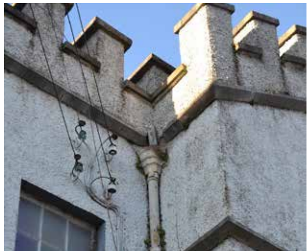
Cast-Iron rain water goods to be labeled, carefully dismantled, repaired, and reinstated
