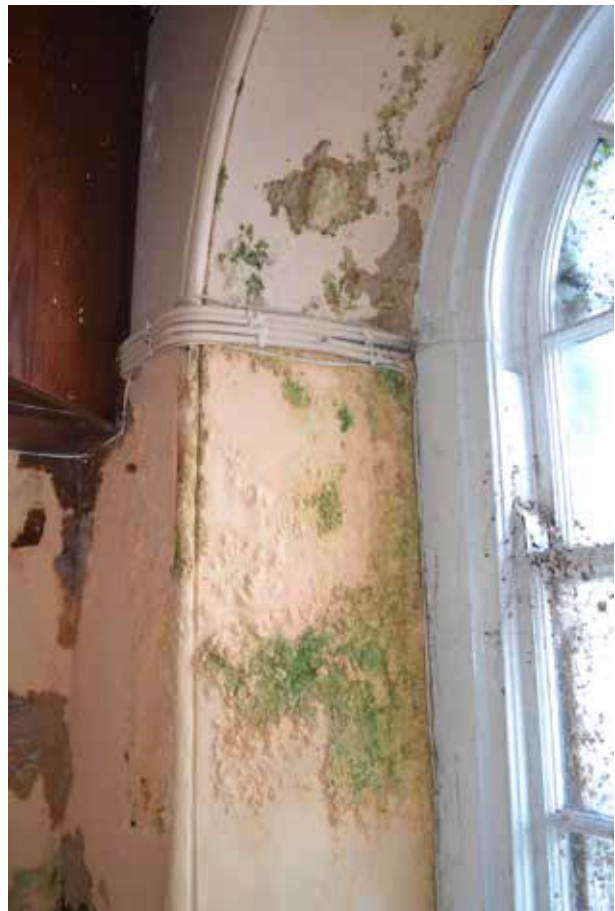
Area A: Mould and bubbling plaster in window reveal on ground floor.
