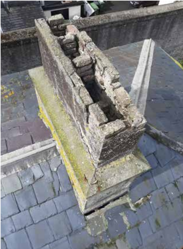
View of the chimney on the west end of the south range roof
