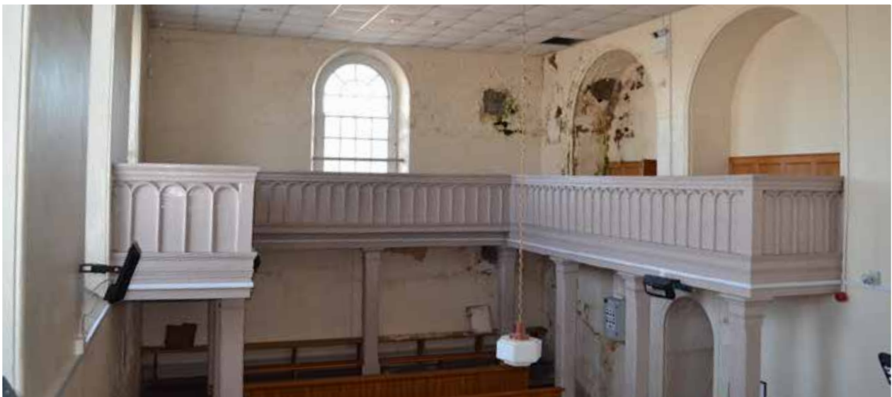
Interior of former courtroom, significant decay visible in corner of timber gallery.
