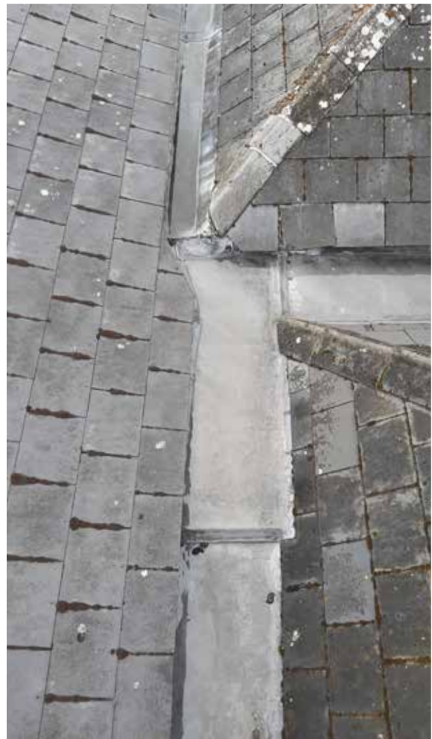
Poorly detailed leadwork - excessive water ingress noted at this location
