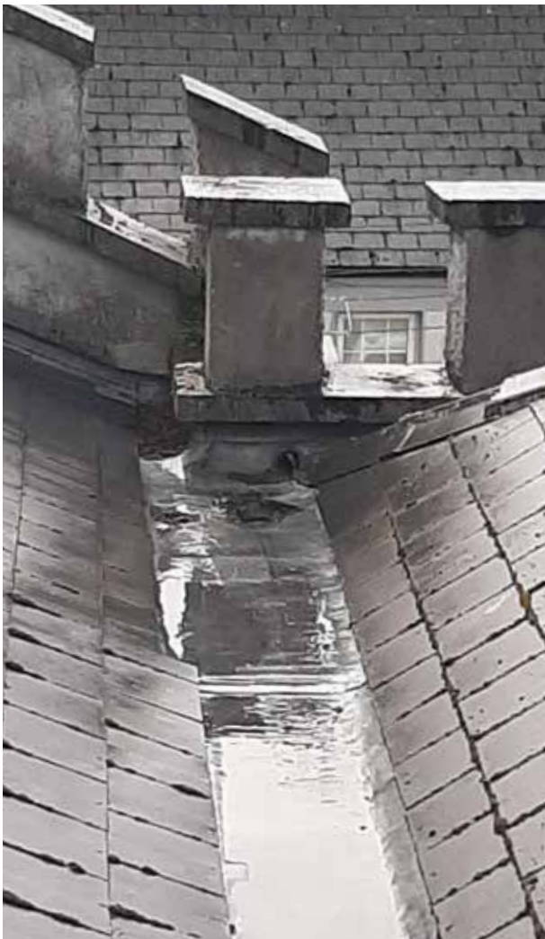
Water ponding on the existing leadwork valleys
