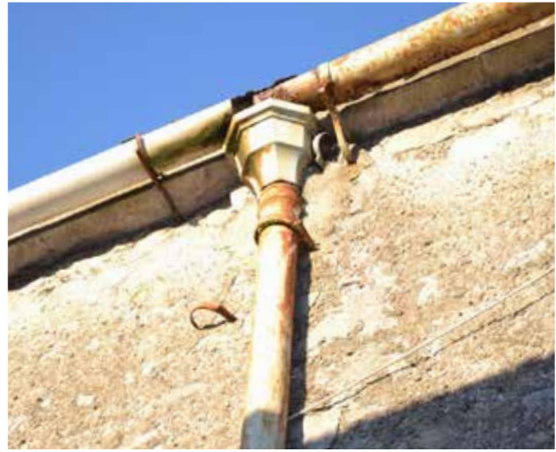
Cast-Iron rain water goods to be labeled, carefully dismantled, repaired, and reinstated
