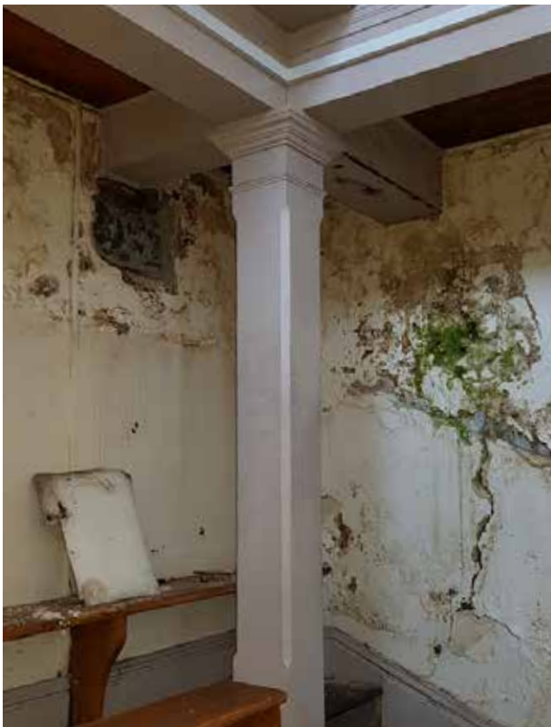
Decay continues below to ground floor level and in direct contact with timber beams. Previous plaster opening up works visible beneath beam of gallery.
