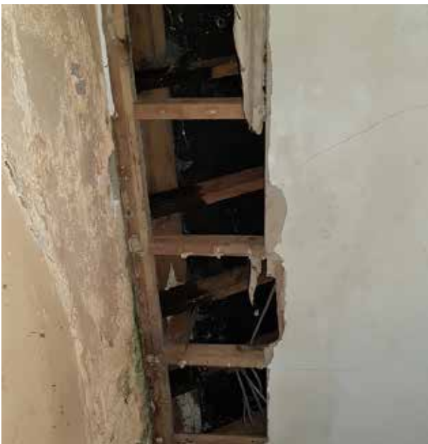
Area D: Collapsed ceiling in stairwell
