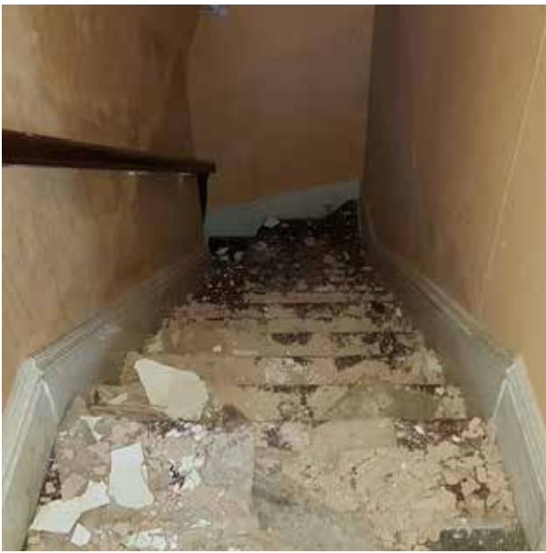
Area D: Collapsed ceiling in stairwell
