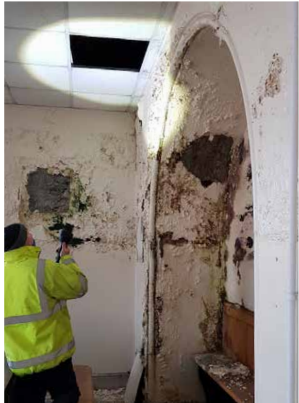
Area of significant decay on corner of courtroom gallery Water ingress and rot in direct contact with joinery
