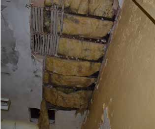
Area B: Collapsed lath and plaster ceiling
