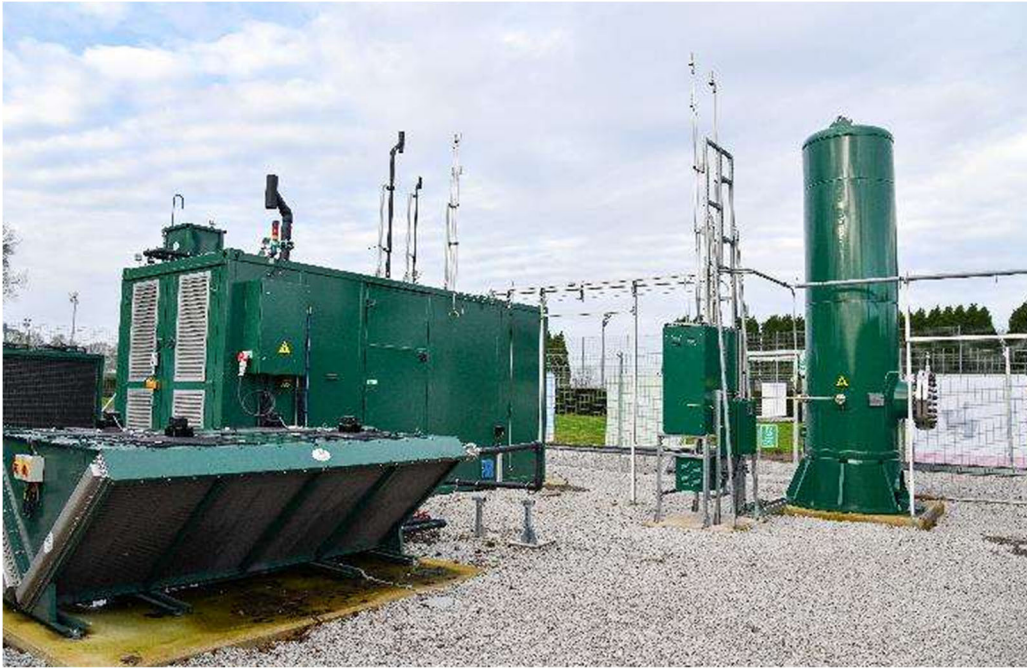
Figure 4-9: HyDeploy Phase 1 0.5MW Electrolyser Installation at Keele University
