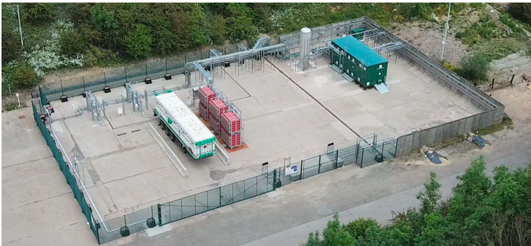
Figure 4-10: HyDeploy Phase 2 at Winlaton (Hydrogen blending and injection only)
