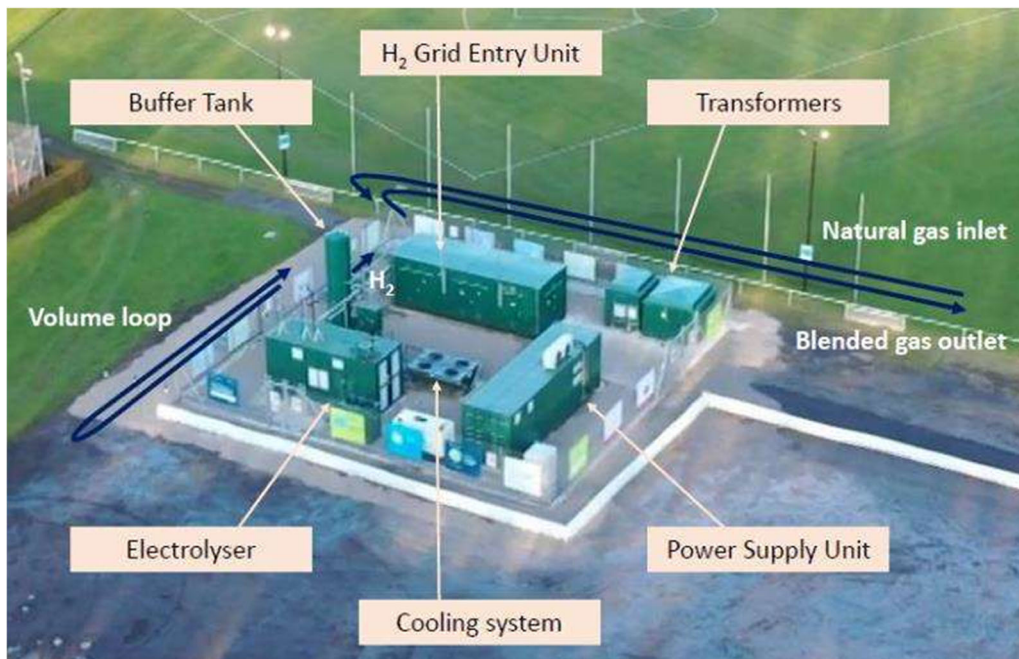
Figure 4-8: HyDeploy Phase 1 trial at Keele University, UK (27)
