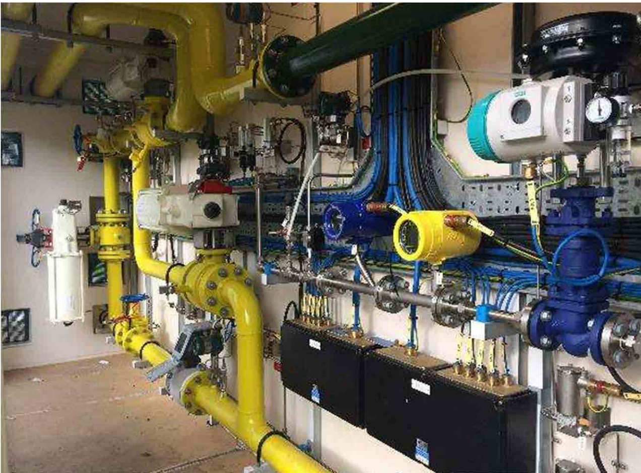
Figure 4-3: Grid Entry Unit used for HyDeploy Phase 1 at Keele University
