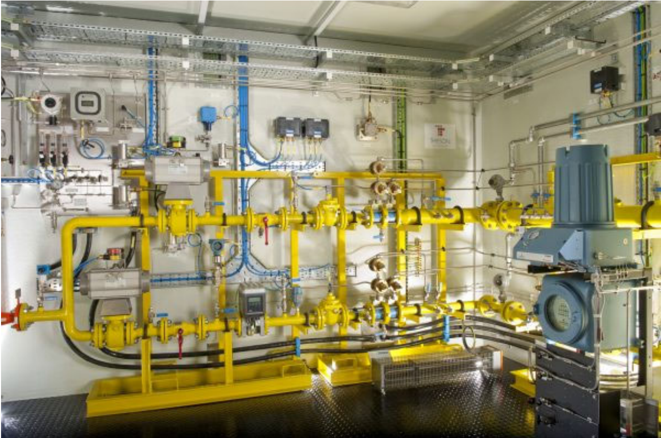
Figure 4-2: Thyson's Propane Vapour Injection equipment coupled with Opto Trim (24)
